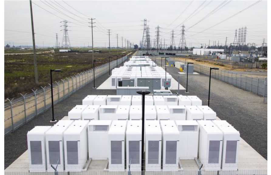
Utility Scale Batteries
